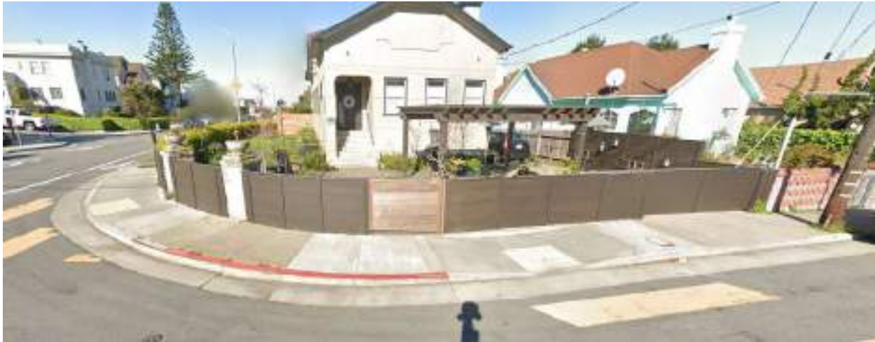
Figure 2. Non-standard curb ramp.
