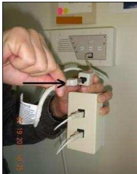
ARROW POINTING TO THE RECEPTACLE
