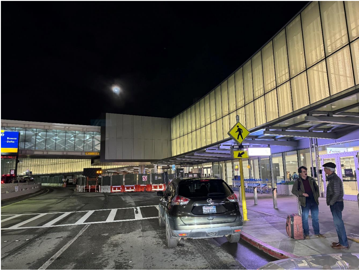
SFO Harvey Milk Terminal 1 - Canopy Glass ABOVE the outriggers - Busy from below where most pedestrians are
