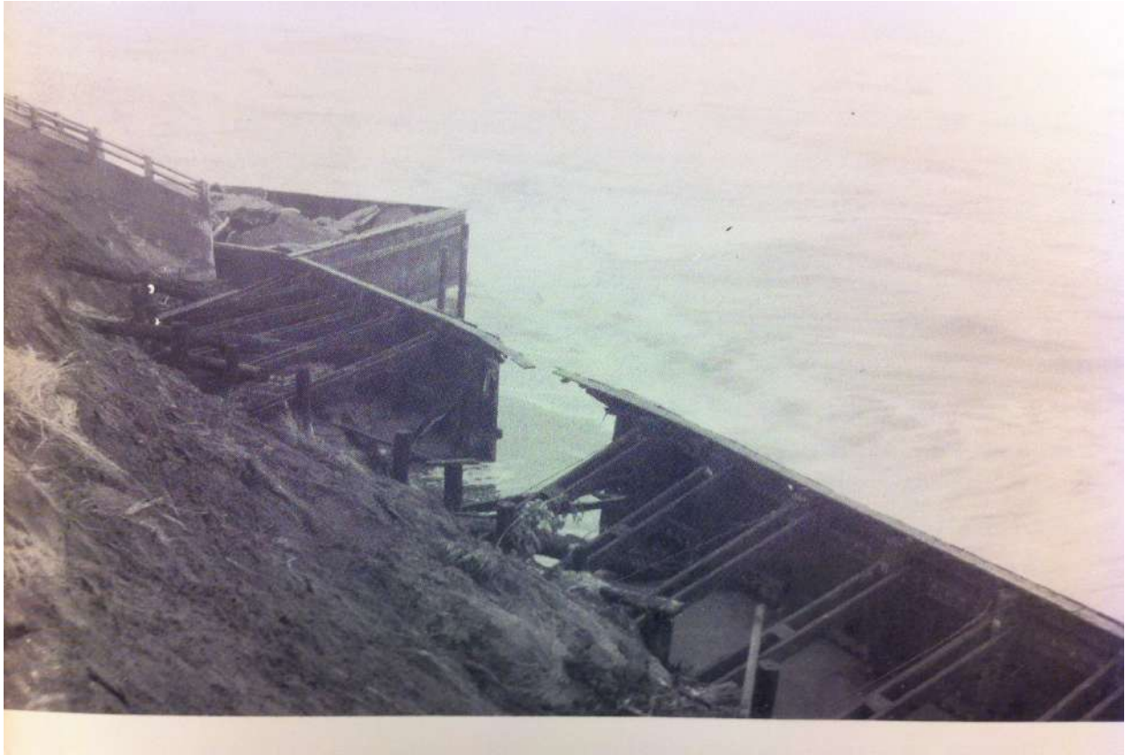
The original seawall at Taraval with storm damage (Olmsted, 1979)
