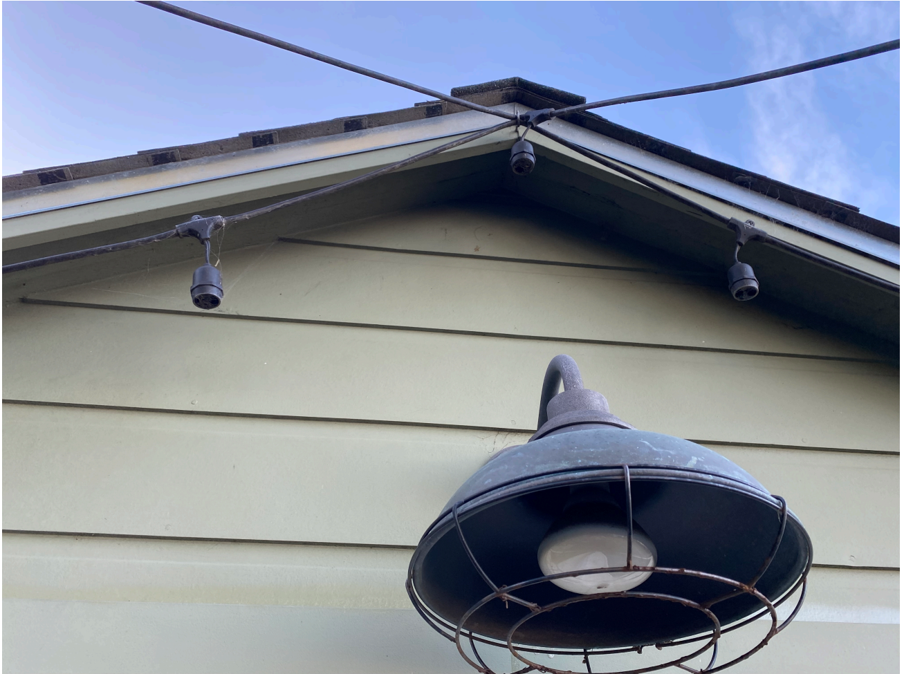
Photo of light bulbs removed from peak of dormer
