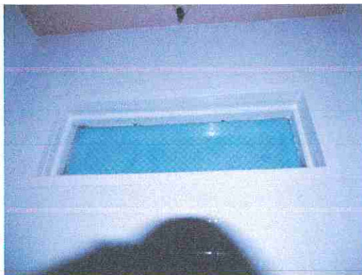
March 4th 2015 Bathroom window covered with blue plastic sheet fixed to outside window Windows in both bathrooms were blocked forcing me to use artificial light
