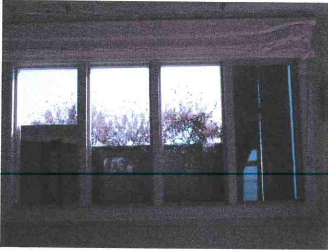
March 31 st 2013 Blocked and Shrubs placed in front of window
