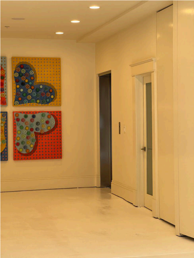
(Item #6) Required door for smoke compartment @ Elevator Shaft:
