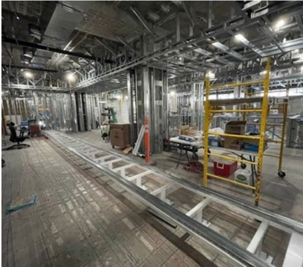
Treatment Equipment Metal Frame Support
