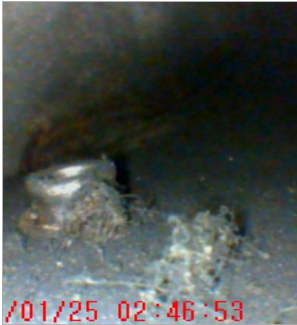
Image 10: During the investigation, conservators employed the use of a boroscope to attempt to confirm connection details and determine statement from the summary documents. Above is an interior view of the pop rivet, ARG/CS January 2023.
