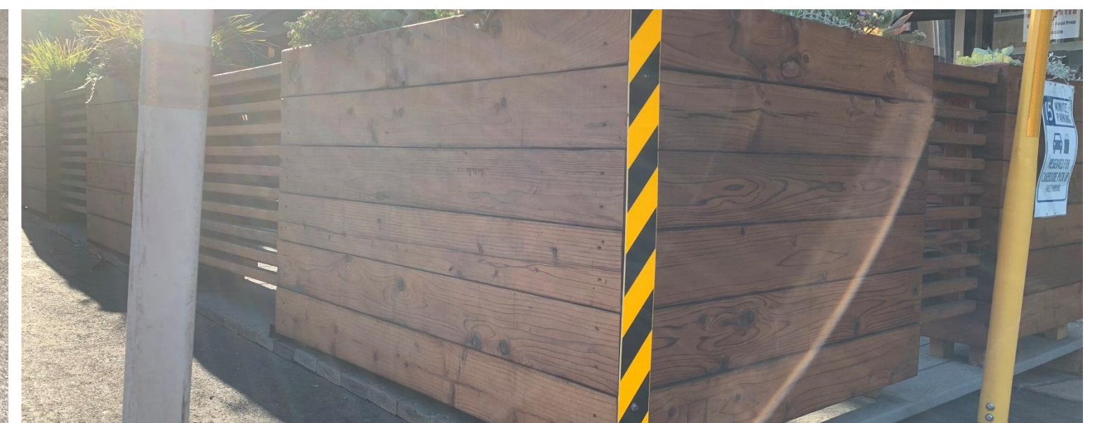
Reflective Materials on Corners
