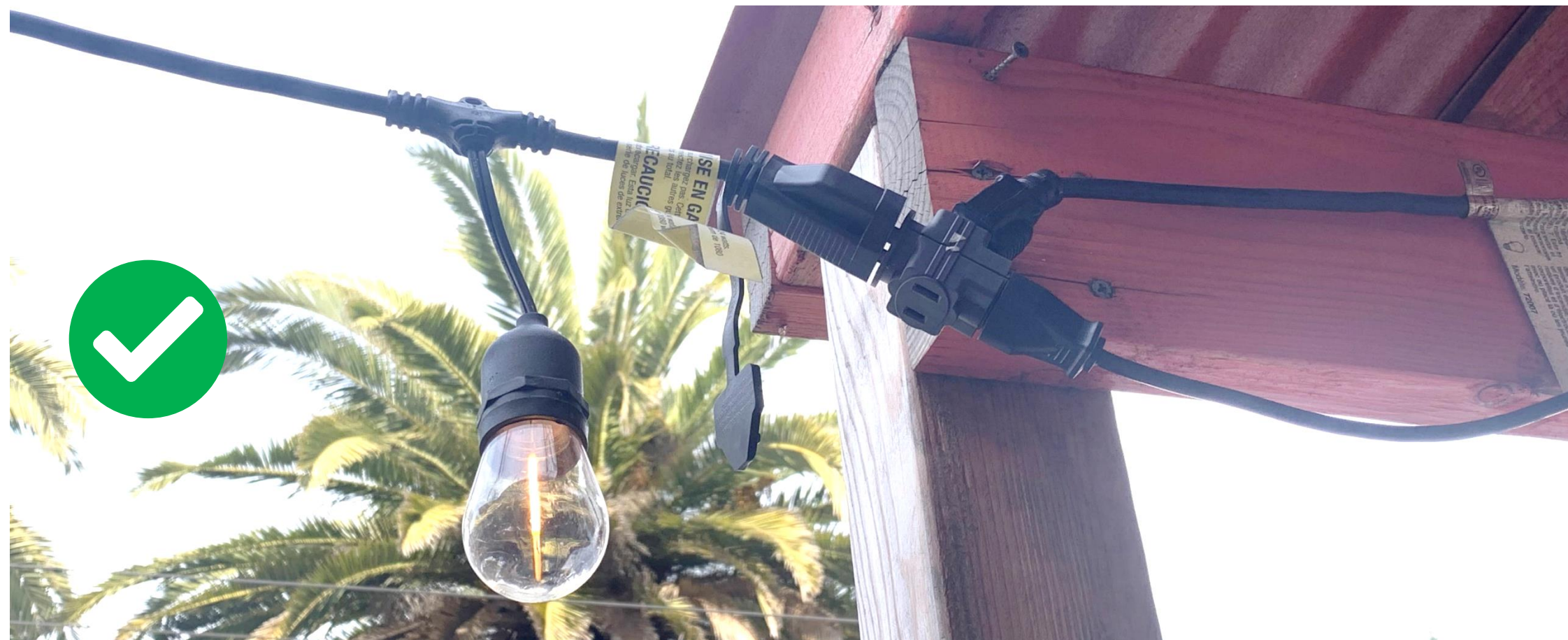
Overhead cables easy to unplug
