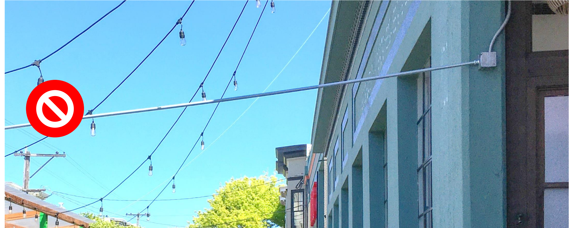
Hardwired connection, or rigid conduit, interferes with ladders
