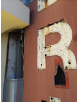
Rusted thru at top of R.jpg 4049K
