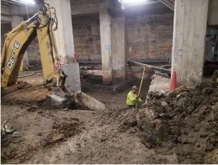
MacArthur Hotel, Los Angeles, CA Project Type: Commercial Earth Shoring Design of earth shoring for deep basement excavation and foundation work for seismic retrofit project.
