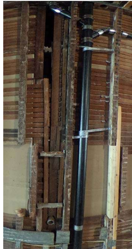
1: New plumbing pipes and electrical installed in party wall without permits
