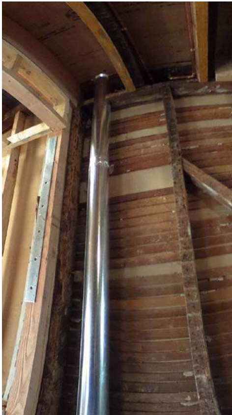
21 22 23 24 25 26 27 28 2: New flue installed in party wall without permits
