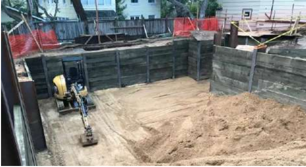
Lincoln Street, Carmel-by-the-Sea, CA Project Type: New Residential Construction Design of temporary earth shoring for basement excavation for new single-family structure.
