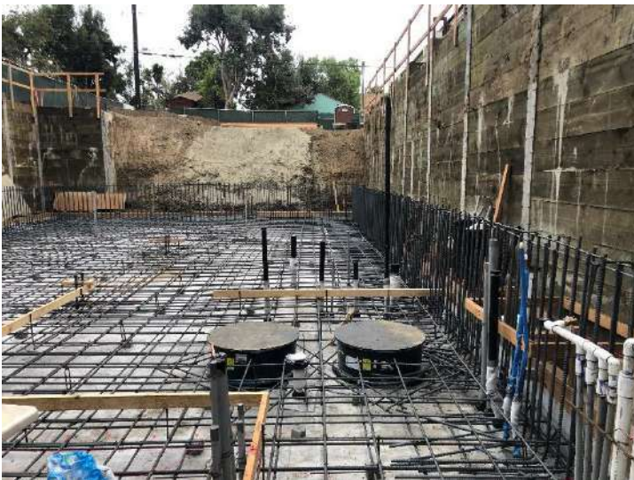
547 7 th Street, Santa Monica, CA Project Type: Residential Earth Shoring Design of earth shoring for basement excavation and foundation work for new residential project.
