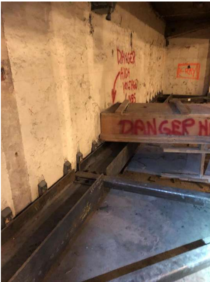
419 South Spring Street, Los Angeles, CA Project Type: Commercial Earth Shoring Basement excavation shoring for seismic retrofit of existing building in Los Angeles. Scope included design of earth shoring, coordination with contractor and various sub-contractors, LADBS and BOE responses.
