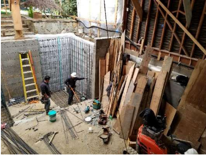
2625 Scott Street, San Francisco, CA Project Type: Residential Construction Design of temporary earth shoring for building excavation, complete foundation installation, and full building renovation. Project shoring consisted of sectional pit construction with concurrent house shoring.
