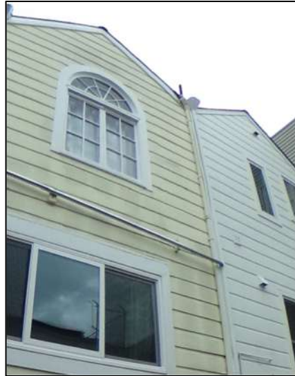
Photo 4: Existing South Face of 1861 Pine Street and 1859 Pine Street (for Reference only)
