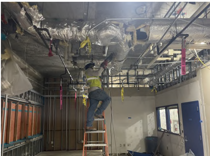
Main Clin Lab – Duct Demo
