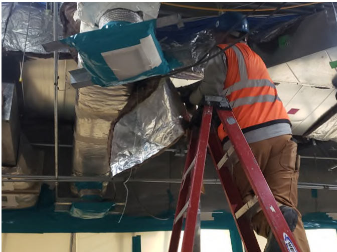
Medical Records – Duct insulation
