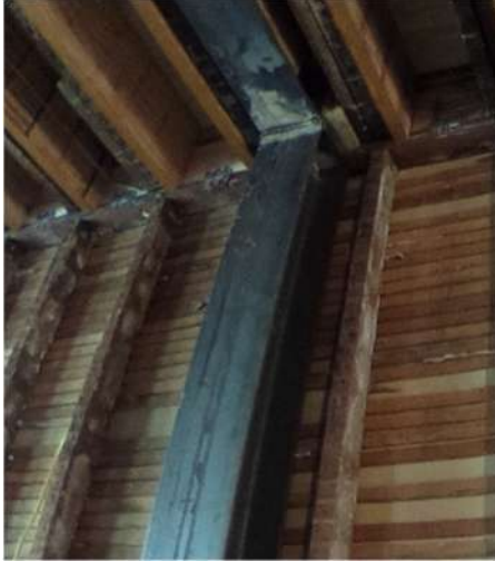
Photo 3: A new Steel Moment Frame Column installed in the plane of the Shared Property Line Bearing Wall
