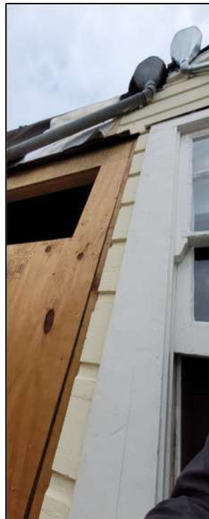
Photo 5: Cut siding at Property Line between 1861 Pine Street and 1863 Pine Street
