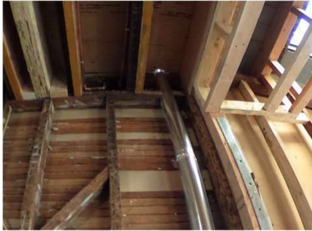
Photo 2: A New Vent Line installed at the Shared Property Line Bearing Wall
