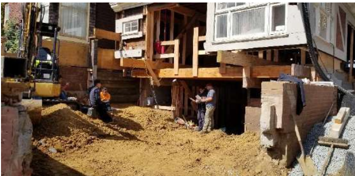
2510 Green Street, San Francisco, CA Project Type: New Residential Design of Residential renovation, addition, and earth shoring. Work included deep foundation work, seismic strengthening, structural renovation and addition, and earth shoring work of Pacific Heights home.
