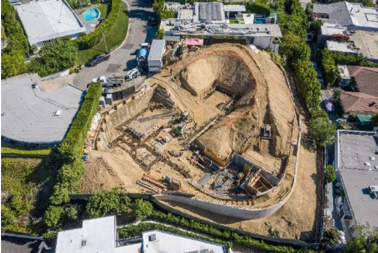
9016 Hopen Place, Los Angeles, CA Project Type: Residential Earth Shoring Design of earth shoring for basement excavation and foundation work for new residential project.
