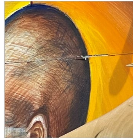
Figure 4: Horizontal cracking of plaster at panel perimeter.
