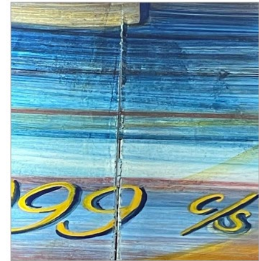
Figure 5: Intersection of four panels where the plaster is cracking.
