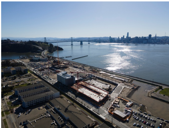
Treasure Island with Star View Court construction in the foreground, image by Andrew Campbell Nelson
